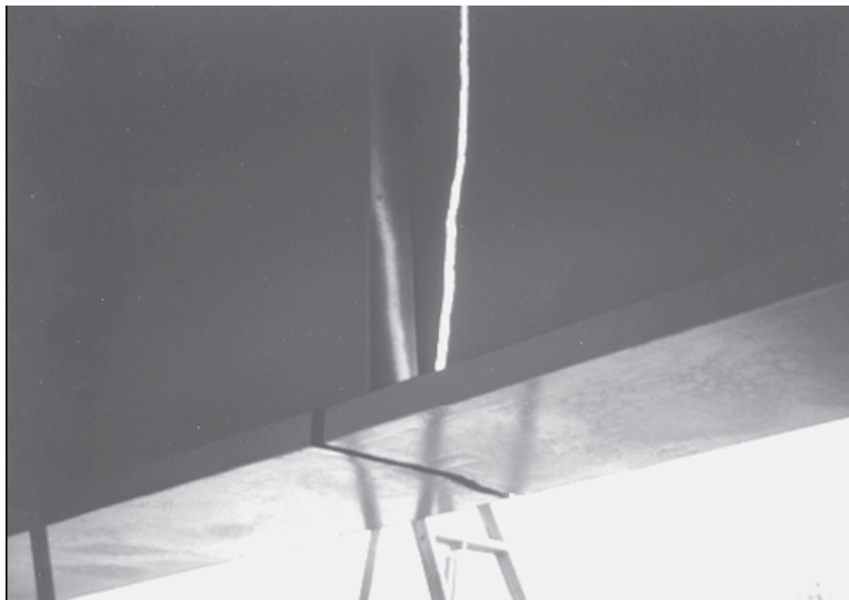
Figure 1.2: Full-depth fracture of the I-79 two girder bridge at Neville Island in Pittsburgh, PA (Connor, Dexter, and Mahmoud, 2005)
